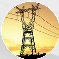
Transmission and distribution overhead lines
